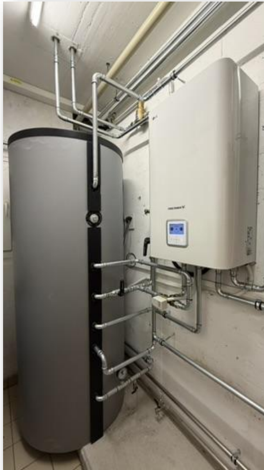
Boiler e centralina
